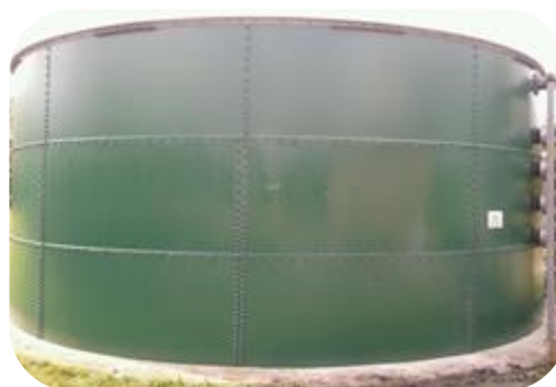
Sectional steel tank containing waste water, abraded mechanically with belt sanders and 2 coats of PES-Chem 508 UVPU applied by roller at 5 mils WFT per coat.
