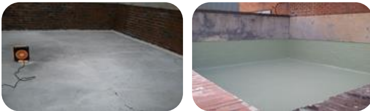
Old diesel bund with concrete floor and brick walls coated with PES-Chem 501 CRSG
