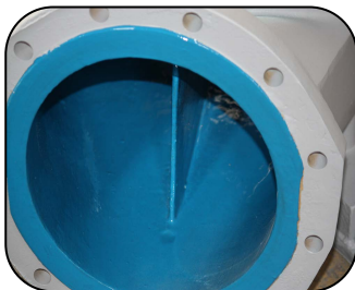
Salt water pump casing
